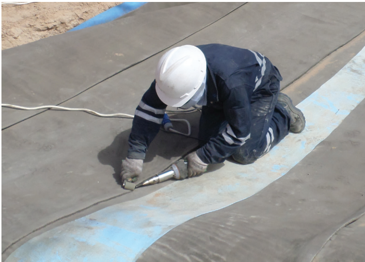
The layers of CCH were jointed using a hot air blower and roller
