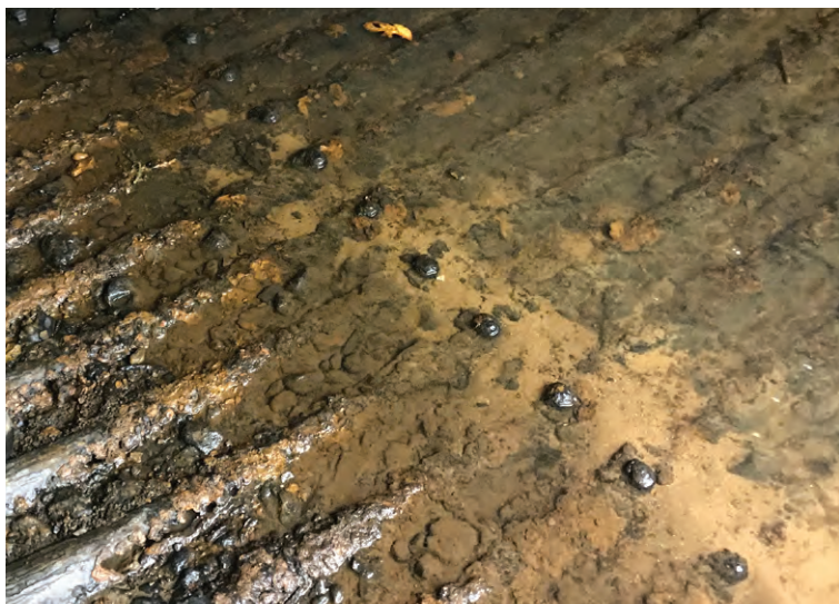
The culvert floor was corroded and heavily sedimented
