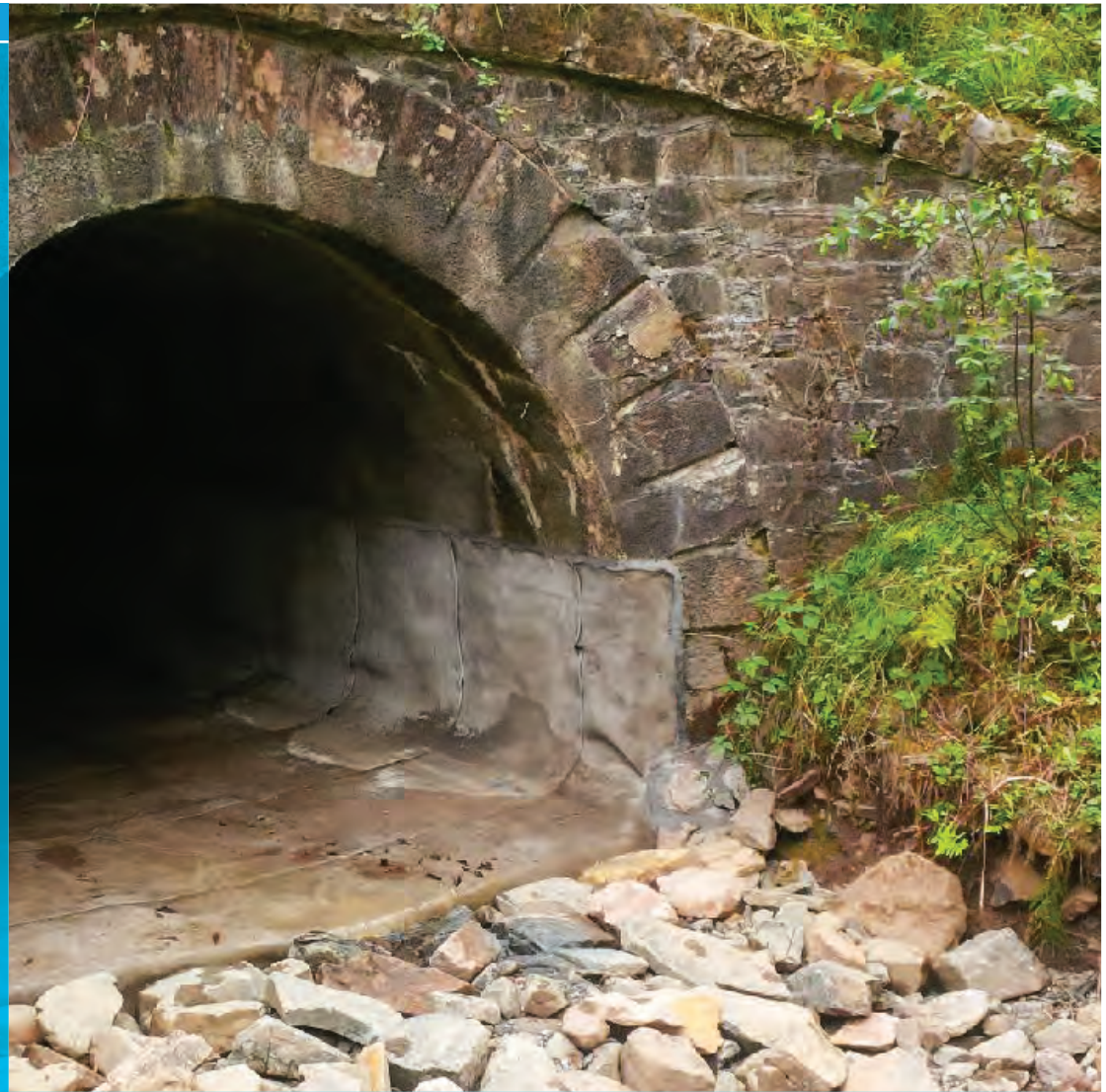
Completed installation in Earlston, Scotland
