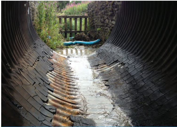
Flow erosion had caused the existing bitumen lining to break down
