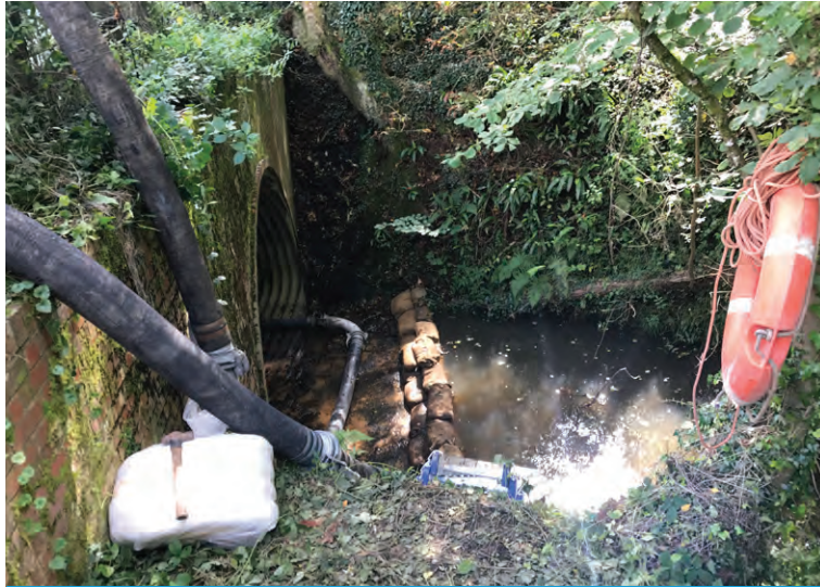
Site access was very restricted
