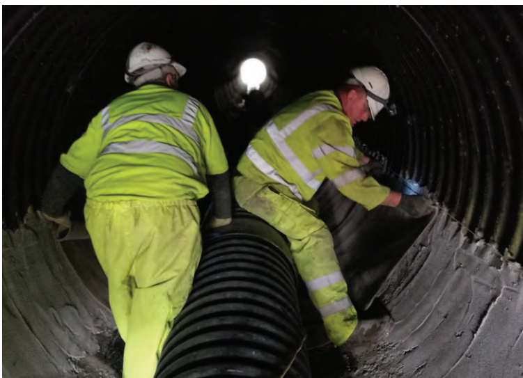
Batched rolls of CC8 were laid transversely across the width of the culvert
