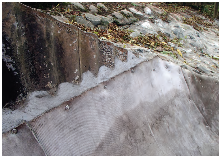
CC was fixed with tech screws & grout applied to prevent water ingress
