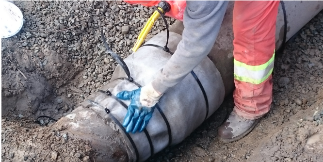
Deltec Cable Strap support used
