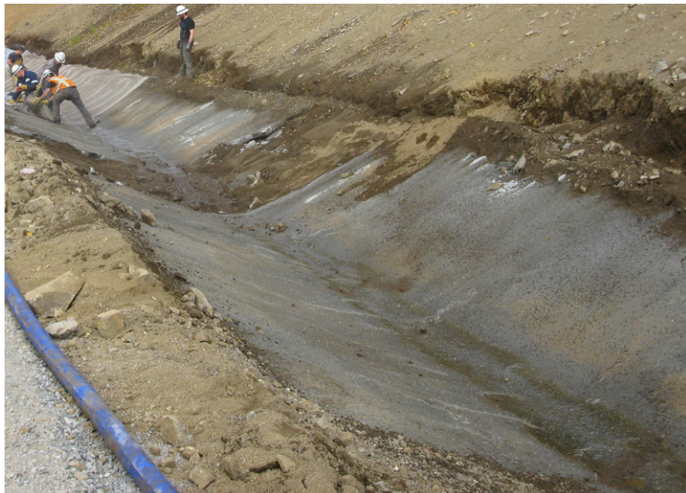
Slope causing the runoff undermining the shotcrete ditch
